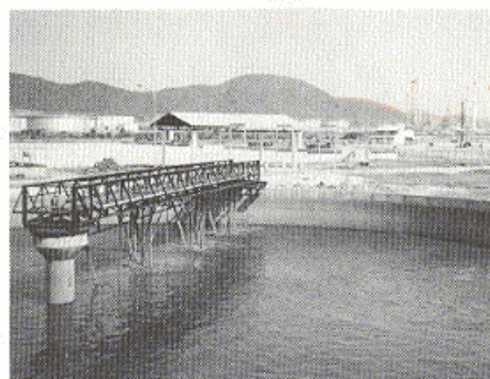
The Laem Chabang Industrial Estate's wastewater treatment plant.
